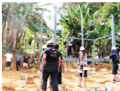
Day 1 - Volunteers listening to the team de-brief and working to put up the steel structure.
