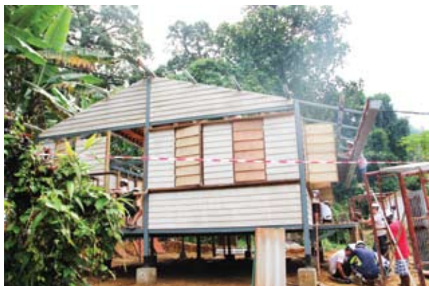
Day 3 - The exterior of the house is up and volunteers are diligently working on the interior.
