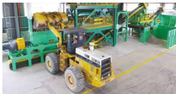
ABS B’s integrated processing line with air pollution control system.
