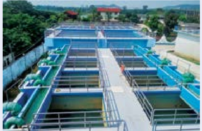
The Pengfa Water Treatment Plant with a production capacity of 30 MLD commenced operations in August 2016.
