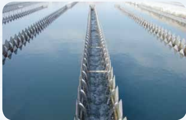
Horizontal sedimentation tank of the surface water plant in Tian Chang City, Anhui Province, People's Republic of China.
