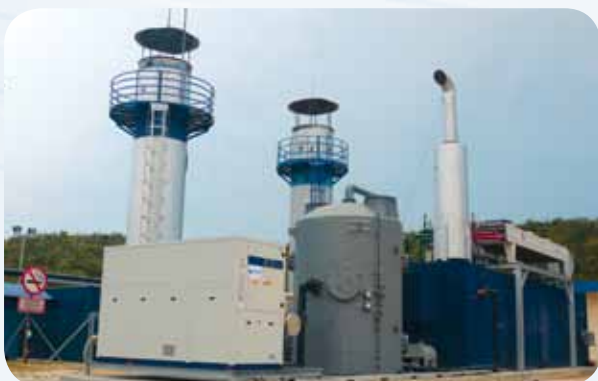
Landfill gas engine and gas treatment system, Bukit Tagar Sanitary Landfill, Selangor.
