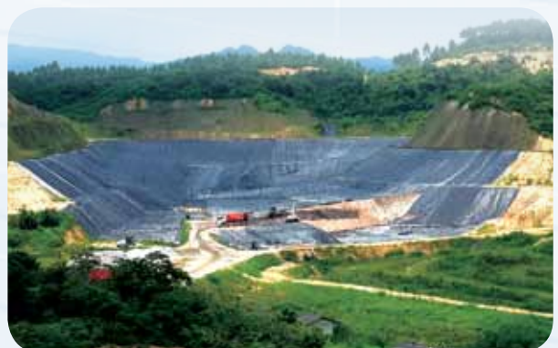
The Sanitary Landfill in Foshan City, Sanshui District, Guangdong Province, People's Republic of China.
