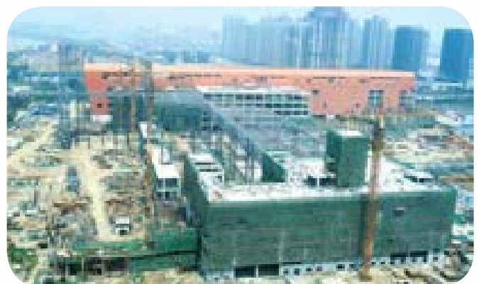
Construction in progress - aerial view of Phase 1 of Great Mall of China.
