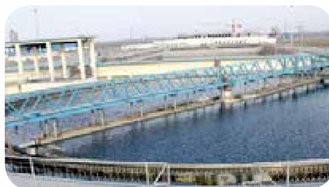
Secondary sedimentation tank – DSG Holdings' water treatment plant in Taian, China.
